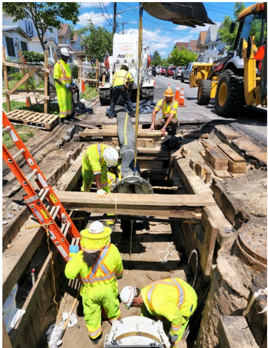
PPM crew prepare the transfer hose for lining the 24" cast iron natural gas pipeline on 134th Street
