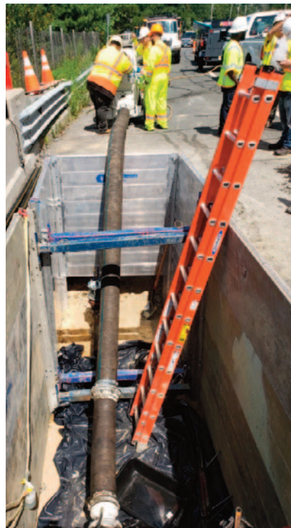
The shoring box used during the project. The shoring boxes are inconvenient as they split the pit into 2 which make it difficult to maneuver personnel and the inversion tube.
