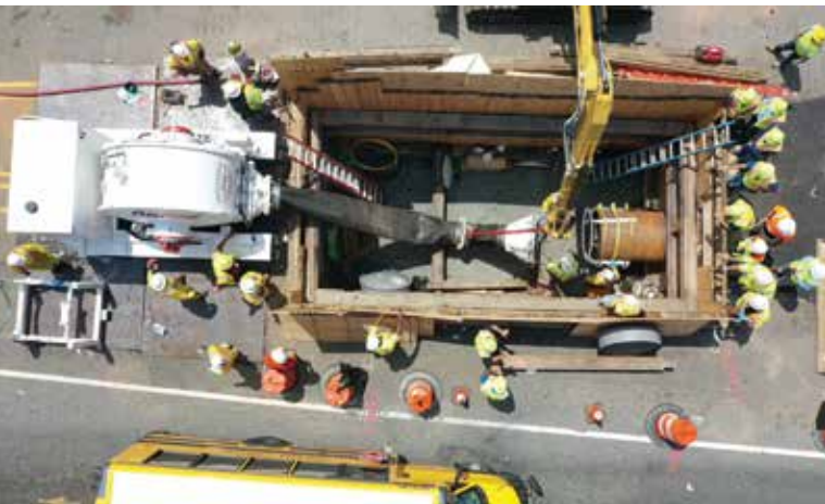
Overhead view of the 42-inch drum, pit and transfer hose
