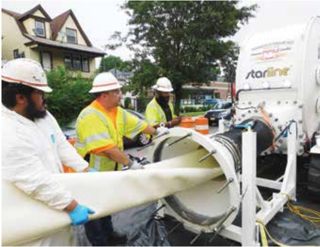
Figure I. PPM team members load the liner into the Starline pressure drum prior to inversion in the excavation pit
