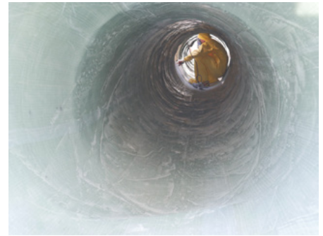
Using confined space entry, the final cured liner was entered to re-instate the center manhole lateral connection
