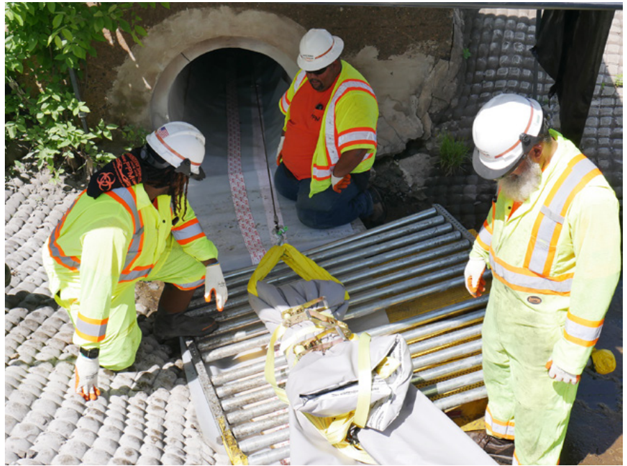
The UV CIPP liner was dragged into place inside the drainpipe using rollers and a winch cable
