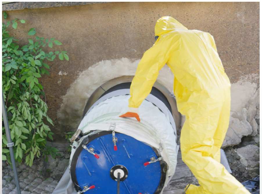
The end gate (blue) had a port on the side for pressurizing with compressed air to inflate the liner. The cable attached was used to pull the liner into place
