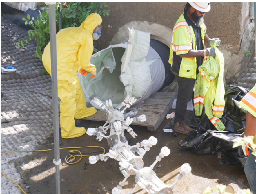
The light chain was pushed and pulled in a timed sequence to cure the inflated liner to the host pipe
