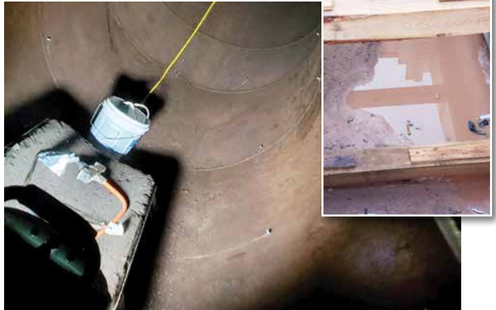
Grout pumped into soil through check valves stopped inflow from heavy rainfall
