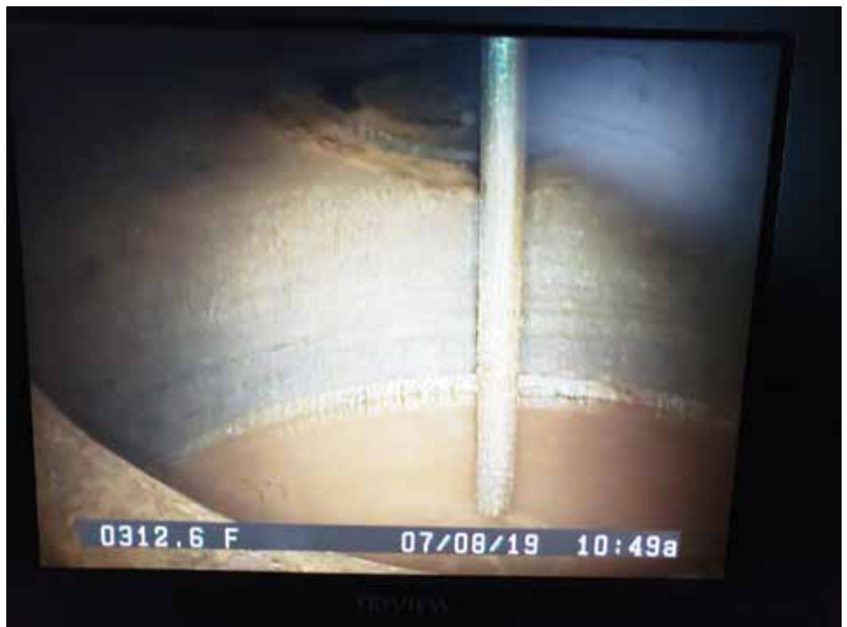
More than 70 gallons of water collected in the drip pot a week after main abandoned
