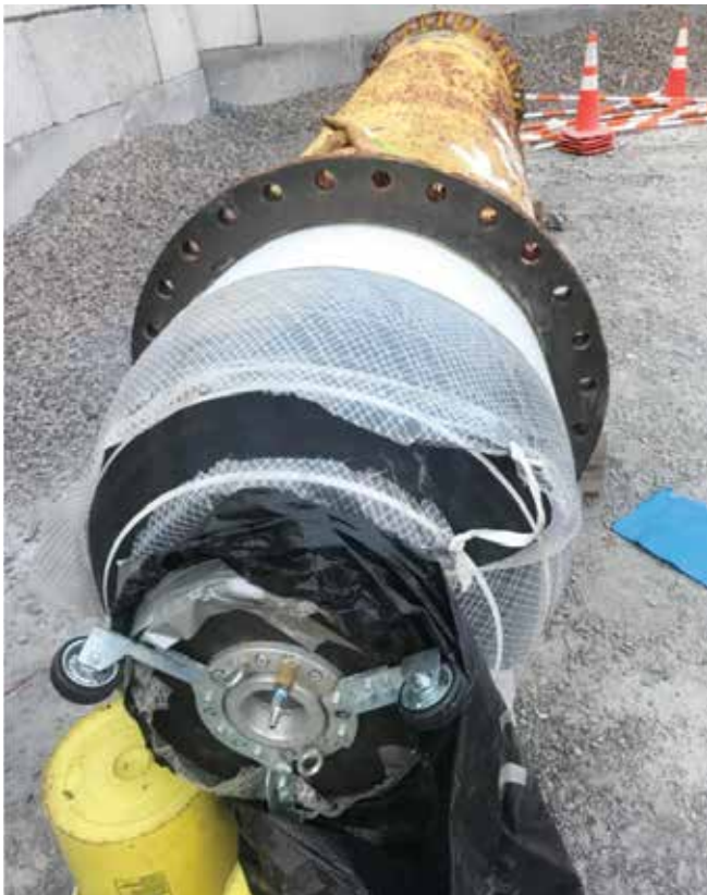
Vertical segment with carbon fiber sleeve that inflates, pushing the liner against the wall of the flange liner to cure and adhere to the pipe wall
