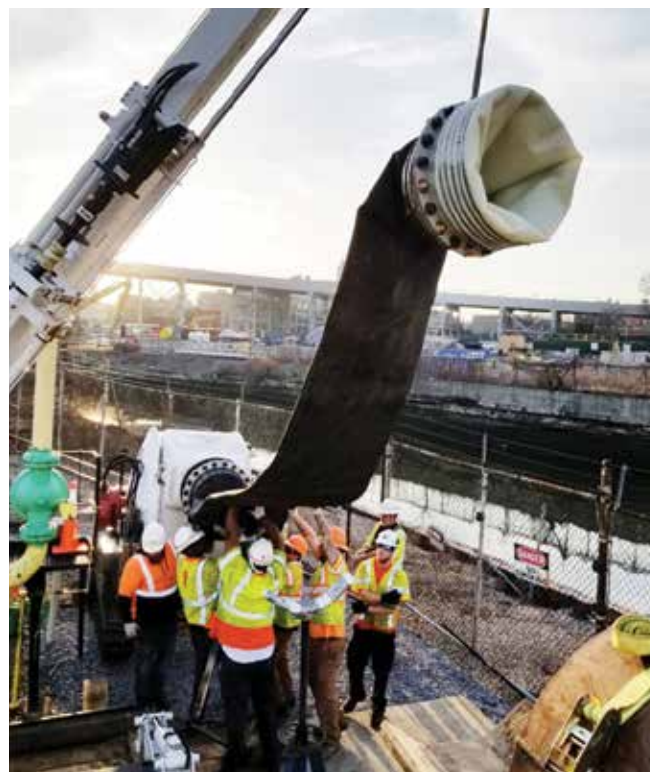
Liner is being inverted as transfer hose is held up by a cherry picker towards the pipeline
