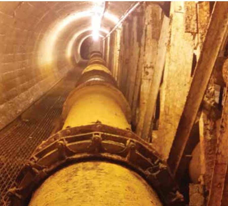
Tunnel underneath Gowanus is over 130 years old. Note the detailed brickwork on the walls
