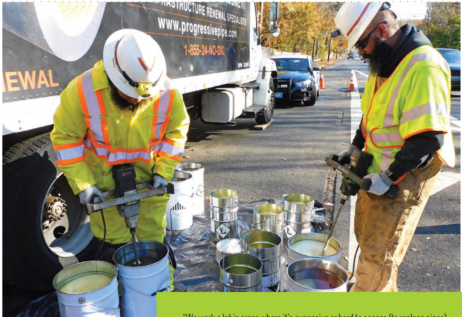
⚡ Miguel Robles (left) and Kacy Wright mix buckets of two-part resin in preparation for lining a 42-inch cast iron host pipe.
