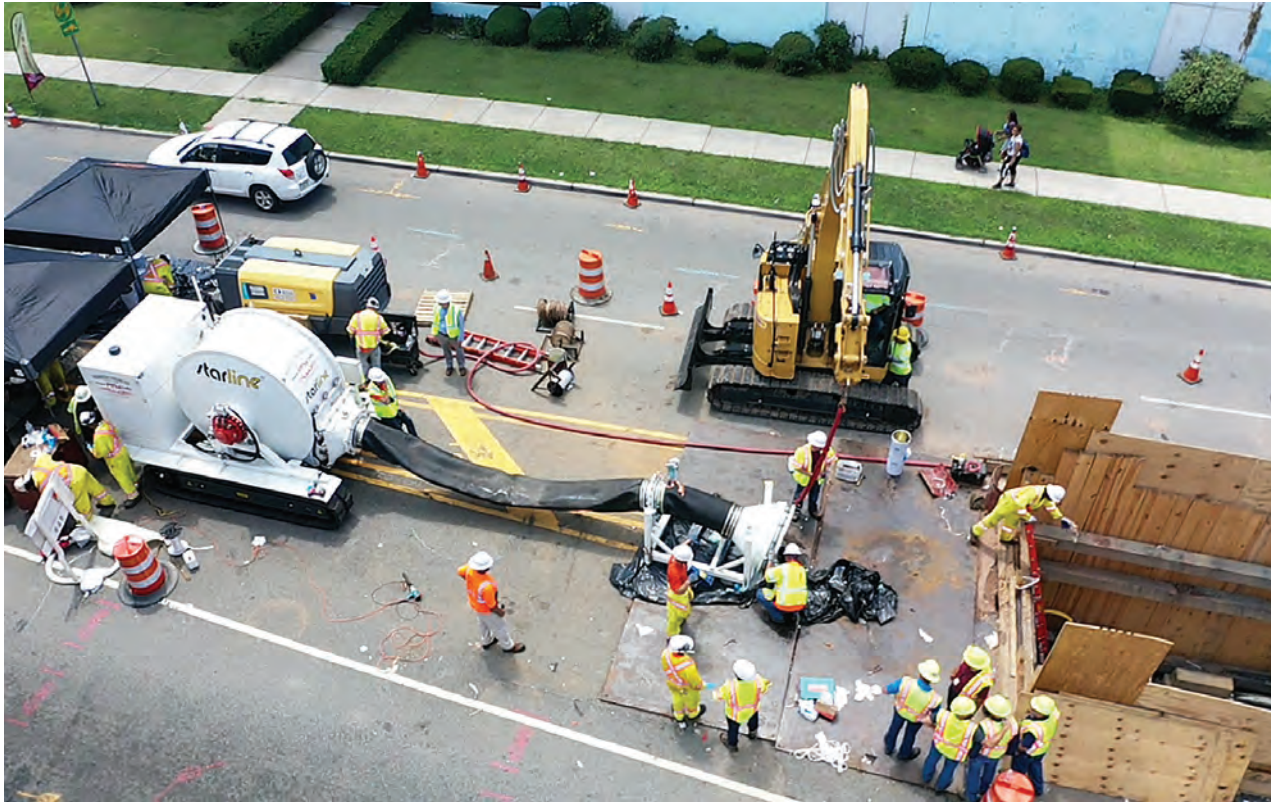
» A bird's-eye view of the PPM crew, starline system and pit during the lining of a 42-inch natural gas main in East Orange, New Jersey.
