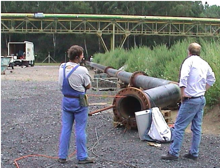
Practical test on Ruhrgas AG premises under supervision of project management witnessing that no blistering occurs with the starline ® 20000 system; 230 ft long test section with pipe expansion and mitered bend in the background.
